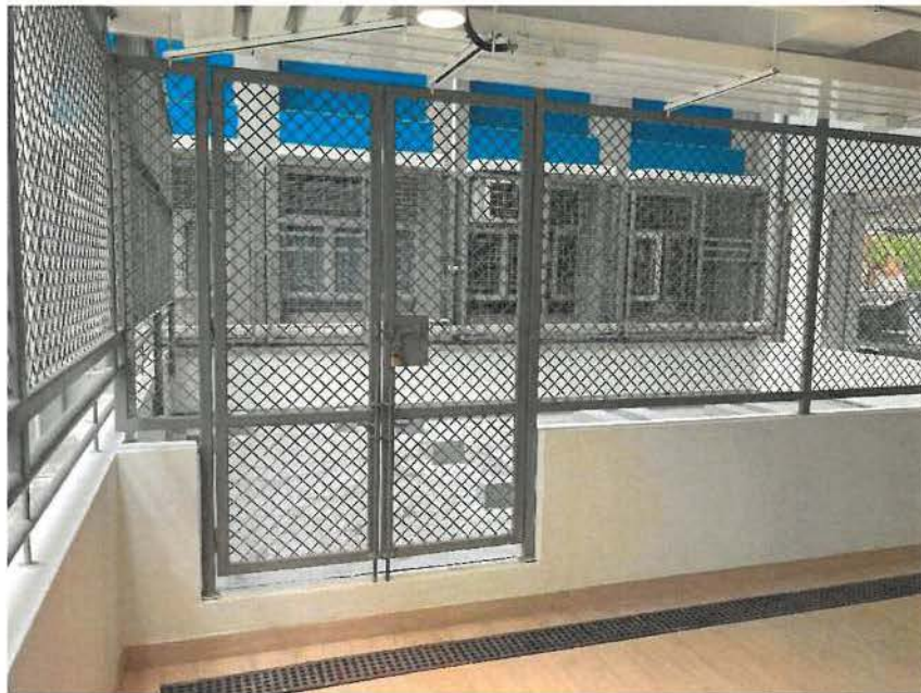
Photo No.: 1-5 Location: A/C platform at 1/F
