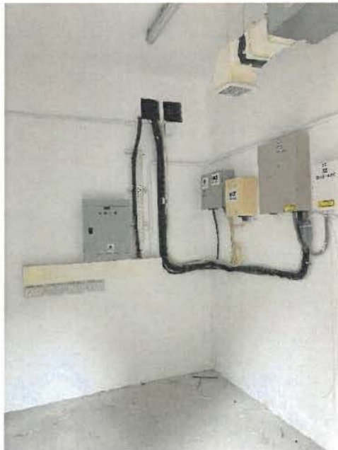
Photo No.: G-8 Location: Telephone and board casting equipment room at G/F
