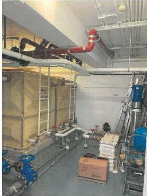
Photo No.: G-5 Location: Flushing water and cleaning water pump room at G/F
